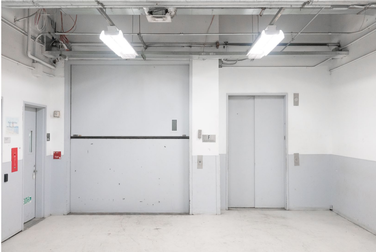
Loading dock freight elevator provides freight access for The Hall and Lower Lobby.
